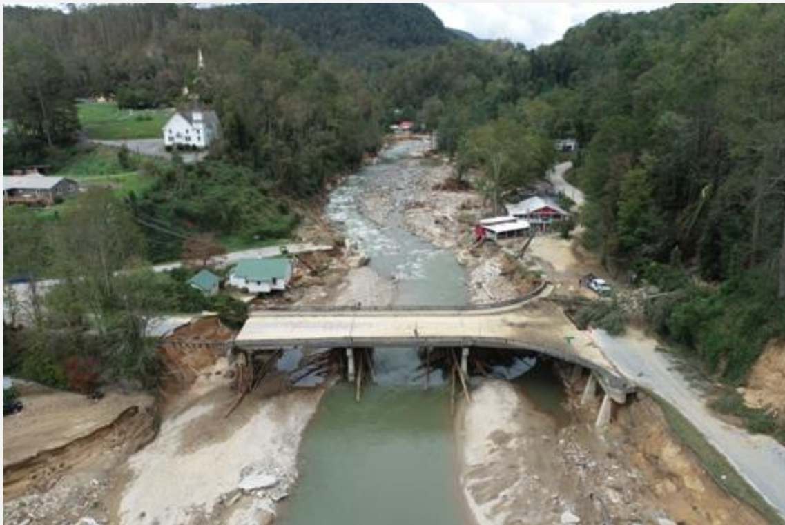
Figure 5: US 64 over Broad River – Hurricane Helene – Bat Cave, NC (September 2024)
