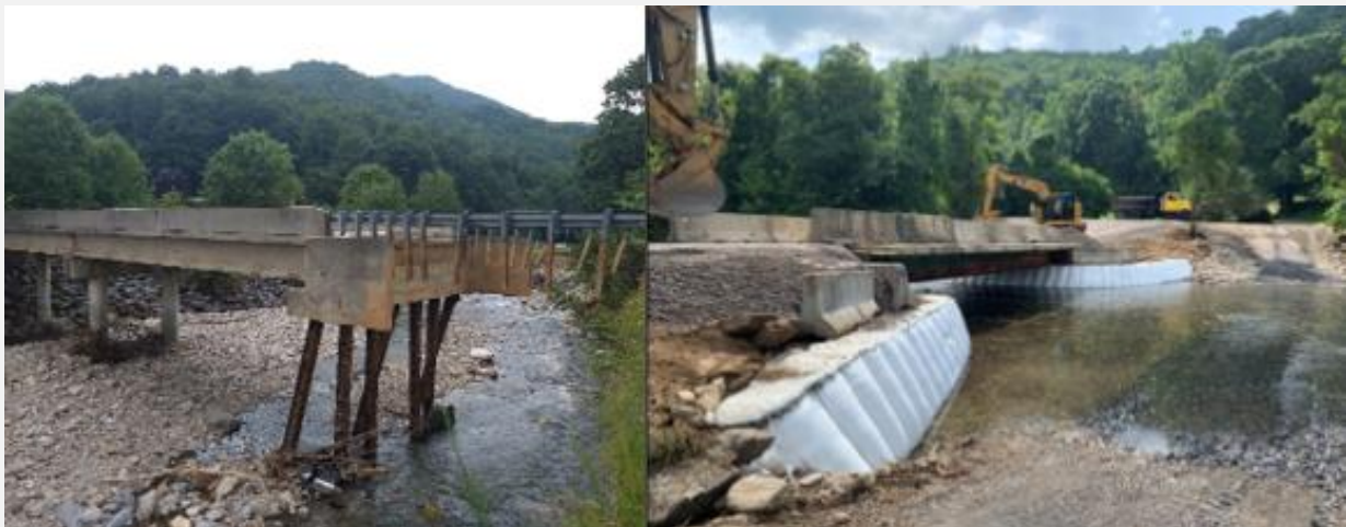
Figure 8: The Closure of a NCDOT Bridge in Yancey County in August of 2021 due to Tropical Storm Fred cutoff a major route in a rural community. Site-specific thresholds like those proposed under NC STRONG were established to monitor the vulnerable temporary bridge during construction.
